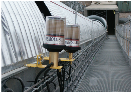
Mineral industry: lubrication of conveyor belt bearings.
