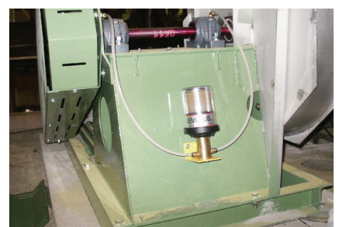
Food industry: lubrication of Solyvent Ventec ventilator bearings.
